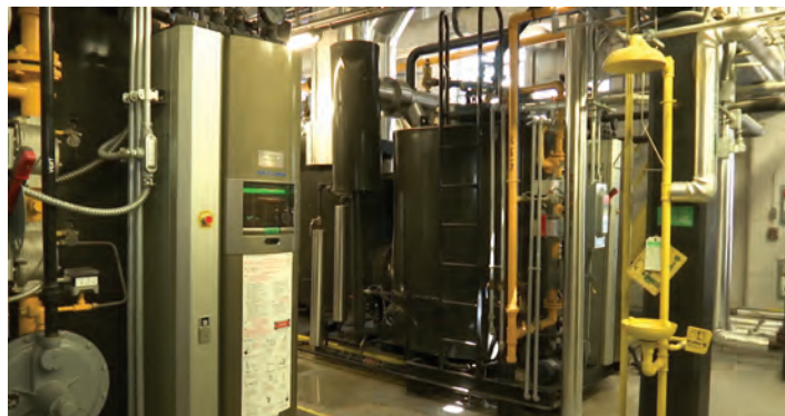
With the assistance of Boiler Masters Inc., Southeastern Health installed four EX-200 SGO Gas/Oil Series High Pressure Steam Boilers in their energy plant and a single 100HP unit in an off-site laundry facility.
